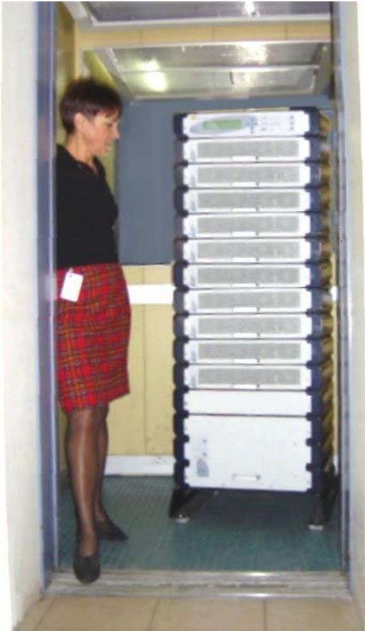
100 kVA – Small enough to fit in a 4-passenger elevator
